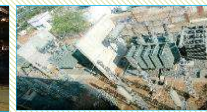
16MVA Transformer (4Nos)
