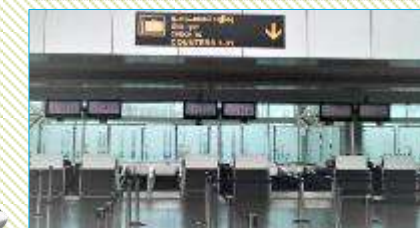
124 'Check - In' Counters
