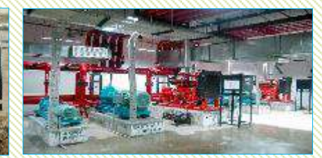
Fire Pump Station
