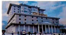
Construction of Auditorium cum Academic Block Building for Srinivasa University at Mangalore, Karnataka.
