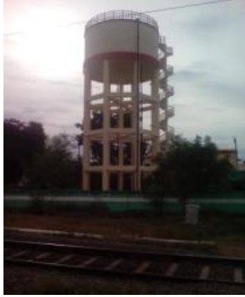
1.40 LL capacity SR at Gandhinagar
