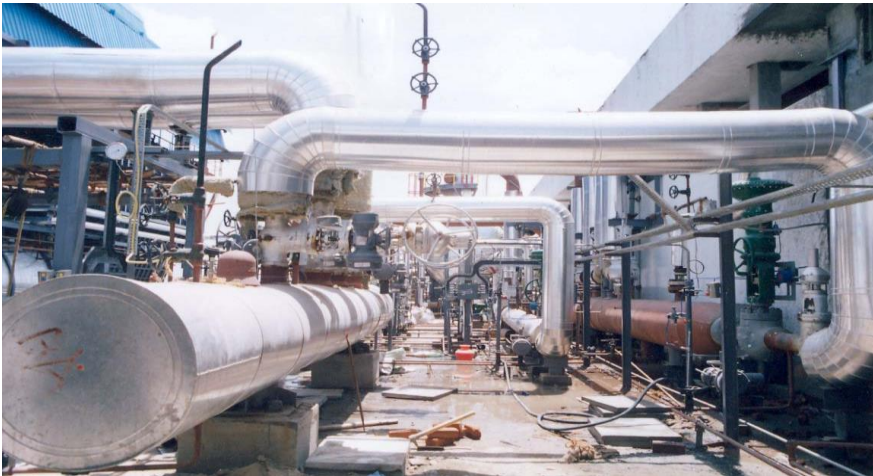
Boilers & Substation Erode (U.G.sump) for Sakthi Sugars Ltd, Aapakudal, Erode
