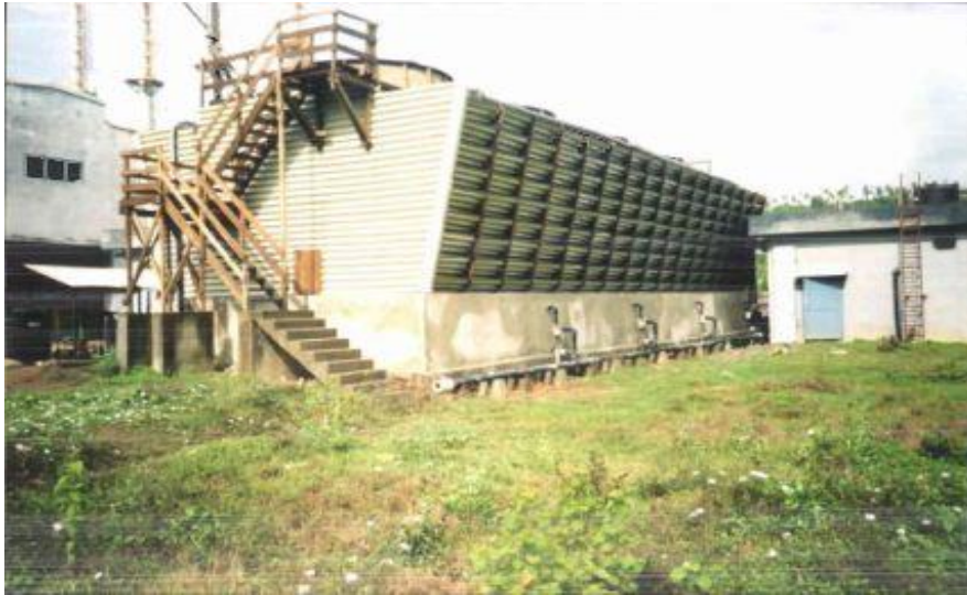
"20MW DG Based Power Plant" for Bses Limited Epc Business Group, Andaman
