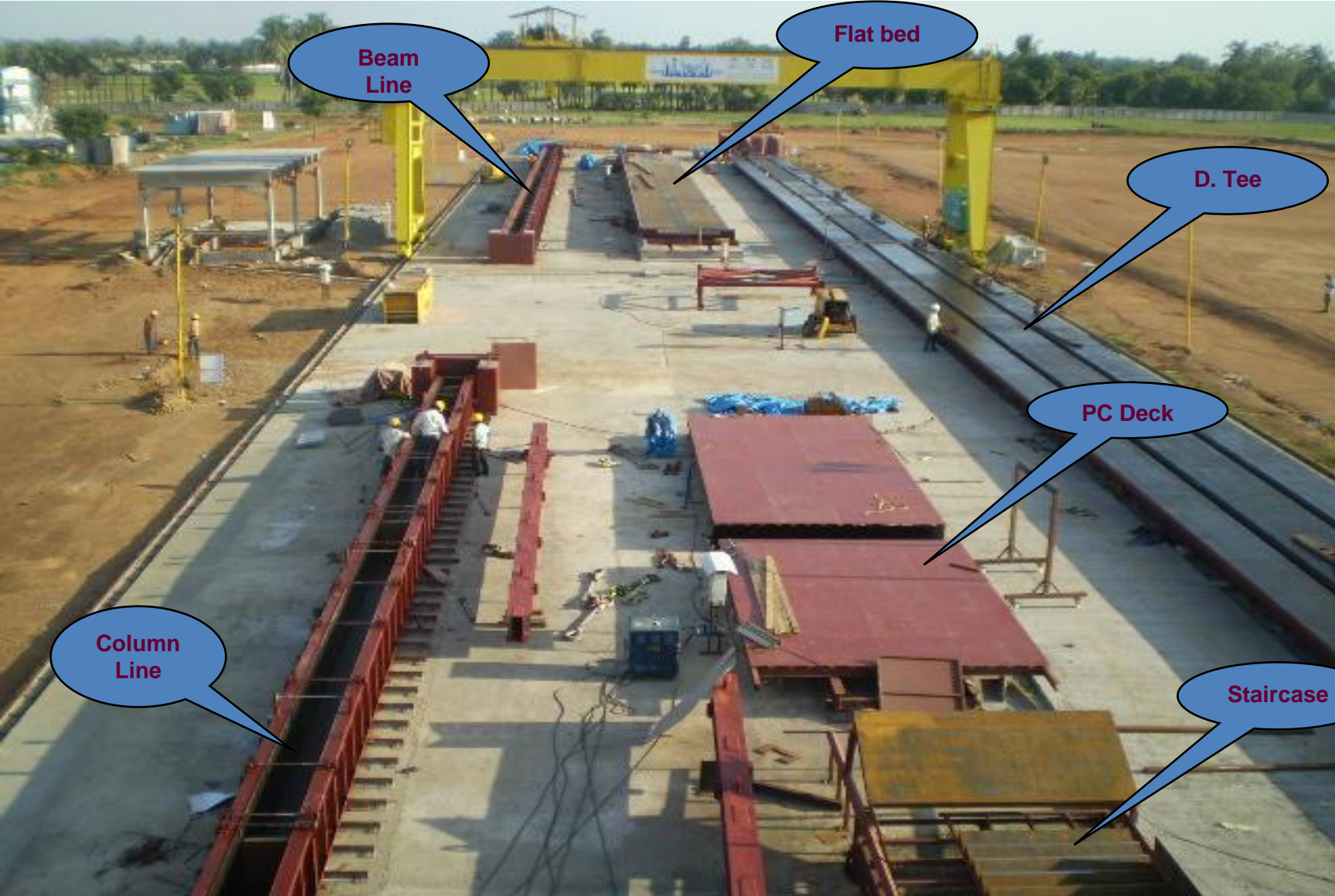
CCCL – C3 – Precast Manufacturing Yard in Chennai (15,00,000Sqft Production Capacity in a Cycle Year)
