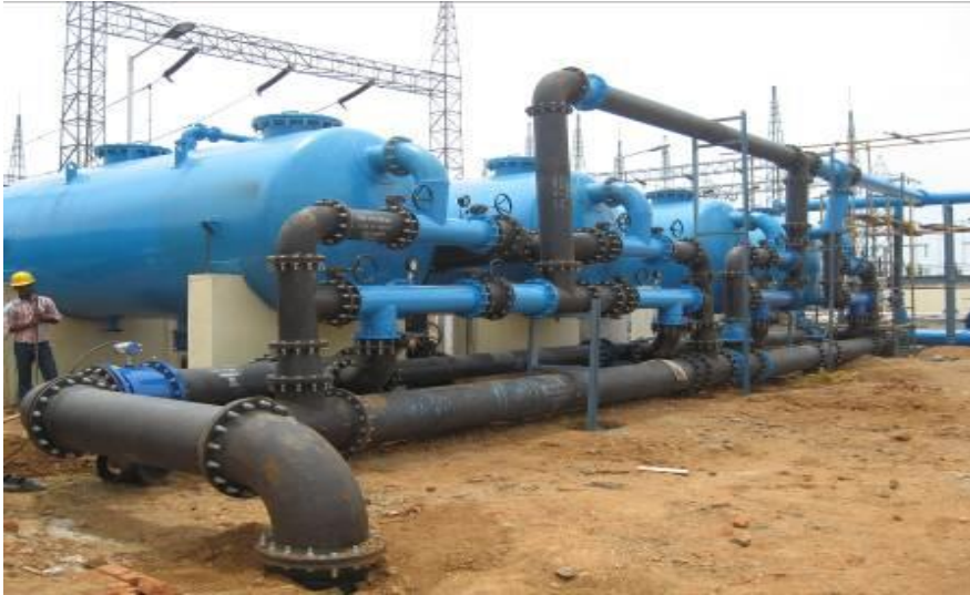
7 MLD Water Treatment Plant, Mahindra & Mahindra Ltd Mahindra world city, Chengalpet, TN
