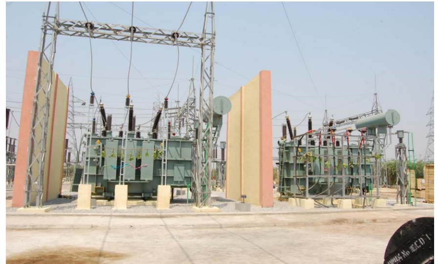
"1X20 MVA, 110/33 KV Tranformer Bay" for Karnataka Power Transmission Corporation Limited, Raichur
