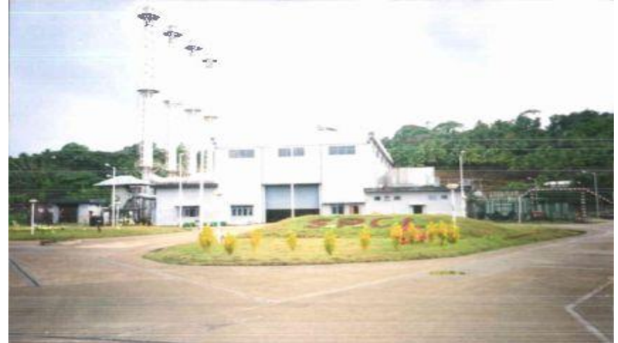
"20MW DG Based Power Plant" for Bses Limited Epc Business Group, Andaman
