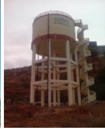
1.70 LL Capacity SR at Veeravanchinagar
