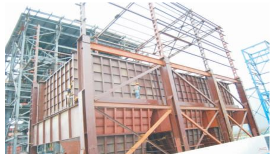
"Coal bunker" for OPG Power Generation Pvt Ltd, Gummidipoondi, Chennai
