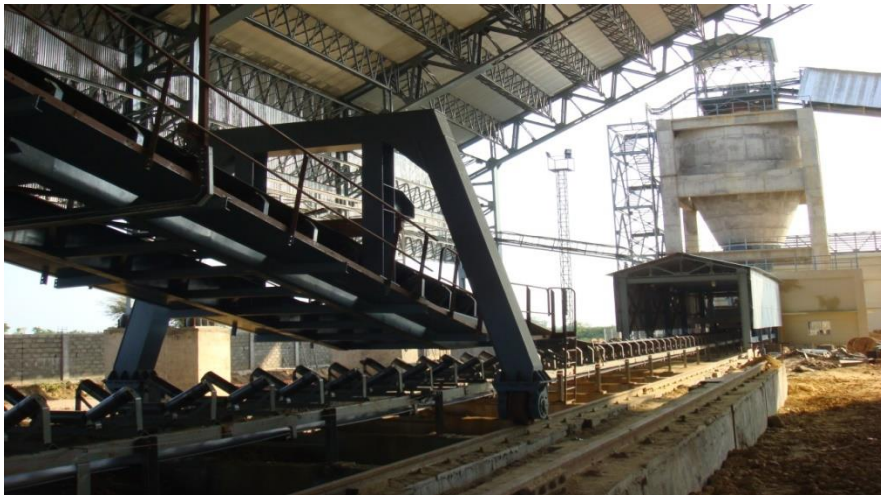
"Surge hopper to lime stone stocker and reclaimed conveyor" for Madras Cements Limited, Ariyalur, Near Perambalur
