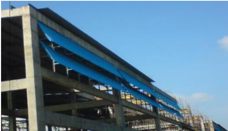
"43 MW Power Plant" for Arasmeta Capitive Power Company (P) Ltd, Chattisgarh,UP
