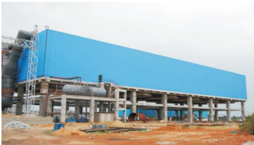
"Air cooled condenser building (ACC)" for OPG Power Generation Pvt Ltd, Gummidipoondi, Chennai
