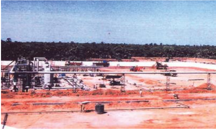
"Gas collection Station" for Southern Petrochemical Industries Corporation Limited ( SPIC - SMO ), Ramanad
