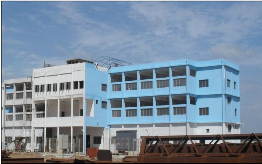
"2 x 500 MW – Compound Wall and Security Office" for Neyveli Lignite Corporation Limited( NLC), Tuticorin
