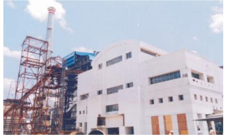
"Co-Generation Power Plant" for Sakthi Sugars Ltd, Appakudal, Erode
