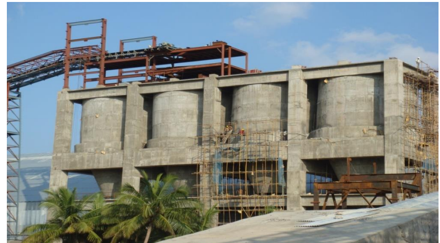
"Lime stone mixing hopper" for Madras Cements Limited, Ariyalur, Near Perambalur
