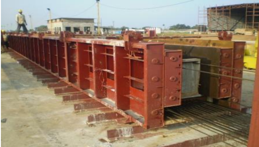
PRODUCTION LINE BEAM
