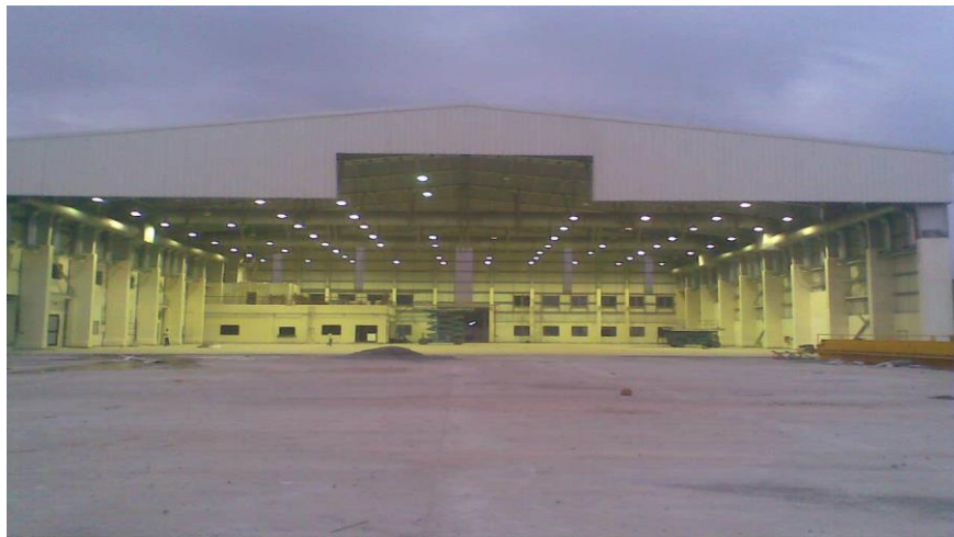
"Construction of Hangars with allied works, adjacent to existing Airport" for National Aviation Company India Ltd (NACIL). Trivandrum Airport, Kerala
