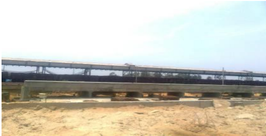
"1x600MW Stage II NCTPS - Pile & Pile cap foundations" for Bharat Heavy Electricals Limited (BHEL), Attipattu, Chennai
